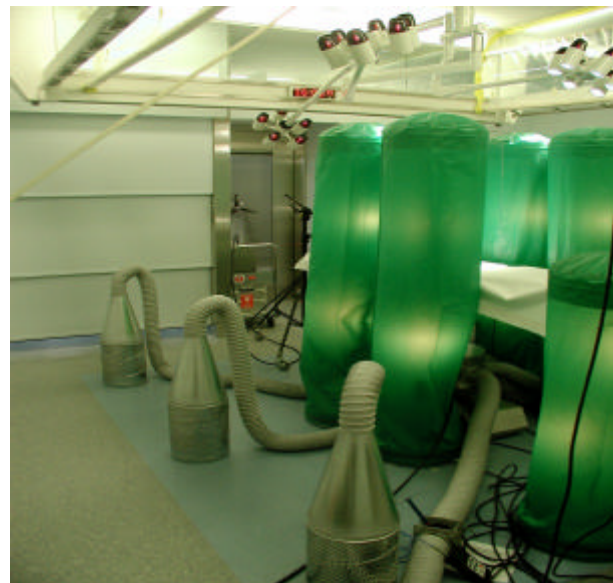
Reference load set-up: Qualification of an operating room GZO-Hospital Wetzikon. A distributor for the reference load is visible underneath the operating table. The sample of air is taken from this distributor for the measurement of particle concentration. In front, the measurement of air velocity for the determination of the volume flow is obvious. This photograph was taken as part of a dissertation. The influence of different diffuser sizes on the degree of protection was aimed to be determined.
