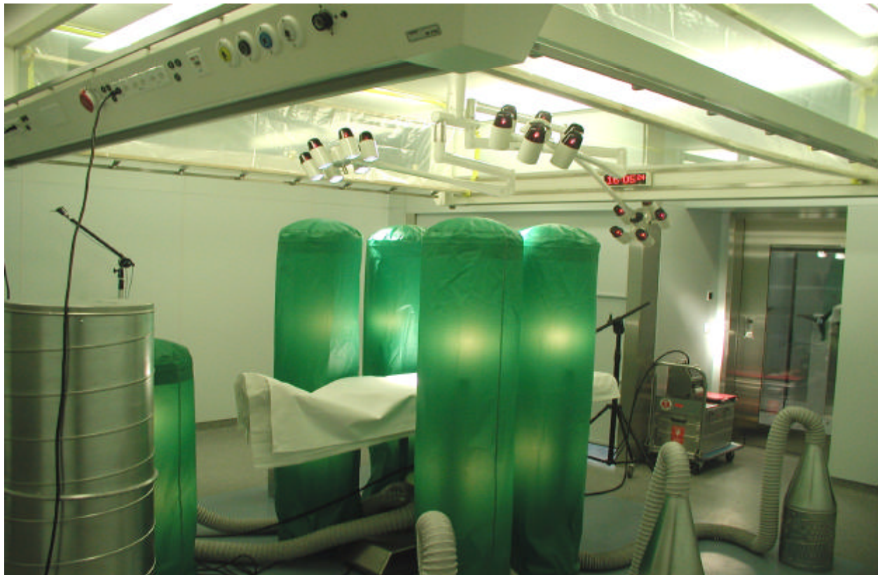
GZO-Hospital Wetzikon (Switzerland) Reference load set-up for the qualification of an operating room
